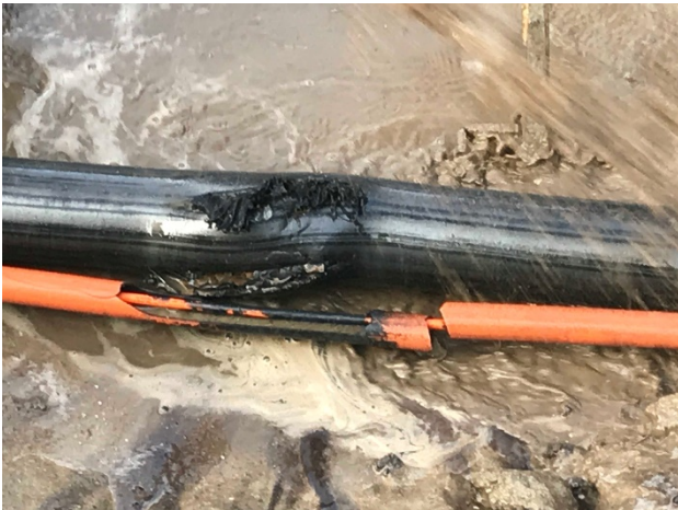
Fig. 11: Fault location. It is clearly seen that the fault was located correctly.
